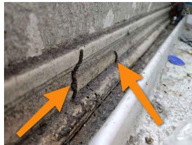
Mud tubes in laundry room behind washing machine
