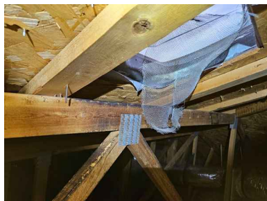
Multiple screens damaged at roof vents in attic area
