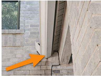
Gutter installed at an angle left of entryway
