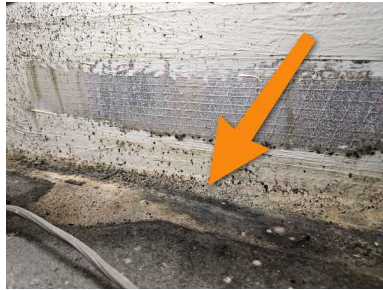
At HVAC closet
