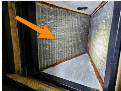
Damaged fins at evaporator coil in HVAC closet - photo 1
