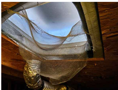
Multiple screens damaged at roof vents in attic area
