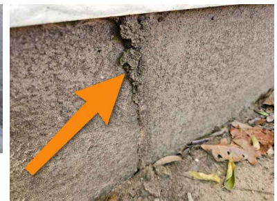
Mud tube at northwest corner of house
