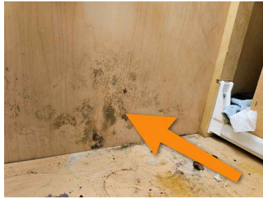
Below downstairs half bathroom sink
