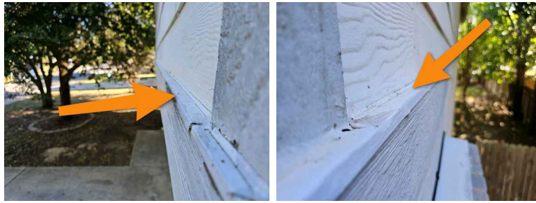
Z flashing negatively sloped at multiple locations
