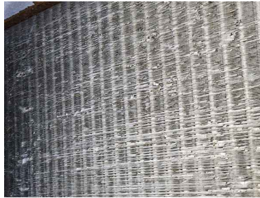
Damaged fins at evaporator coil in HVAC closet - photo 2
