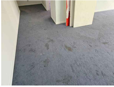
Staining throughout upstairs carpeting material
