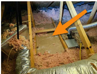
Exposed drywall at various locations in attic area
