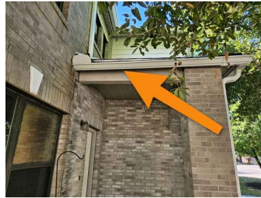
Gutter improperly sloped at front of house
