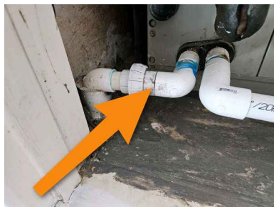
At HVAC closet
