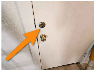
Deadbolt at door to garage
