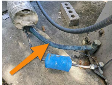
Insulation not present at suction line near condenser unit
