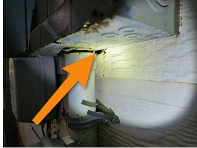
Northwest corner of house below main electrical panel
