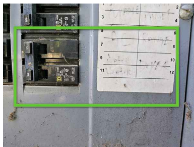
Breaker for dryer at main panel
