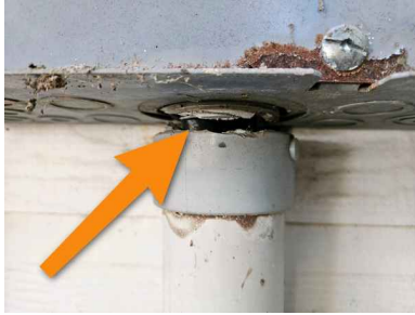
Damaged conduit below main panel for service entrance cables
