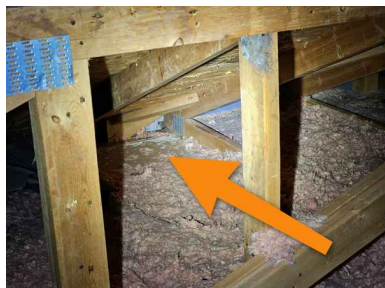
Exposed drywall at various locations in attic area
