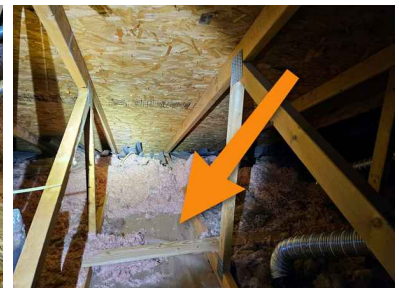
Exposed drywall at various locations in attic area
