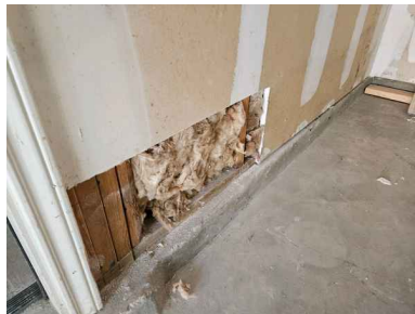
Various locations in garage
