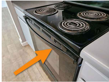
Handle loosely installed at oven
