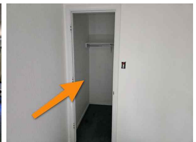
Closet door at upstairs bedroom at southwest corner of house
