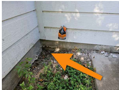
Back of house near condenser unit
