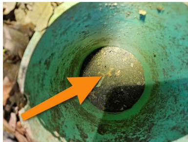
Near water meter
