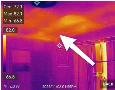
Above bedroom at northwest corner of house - thermal imaging
