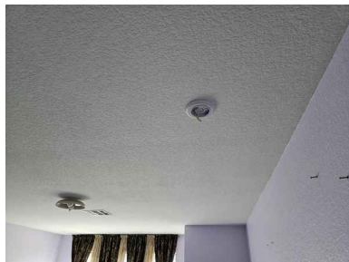
Multiple smoke alarms missing
