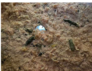
Animal droppings at various locations in attic area
