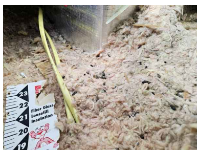
Rodent droppings at various locations in attic area
