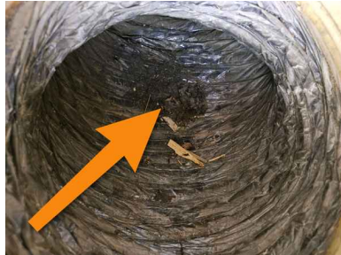
Debris at return ducting below HVAC unit
