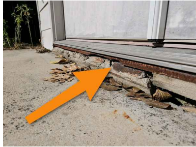
Threshold support below back door
