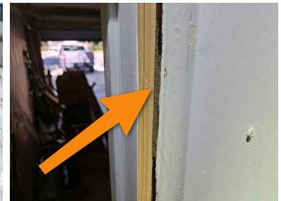
Mud tubes in wall at water heater closet
