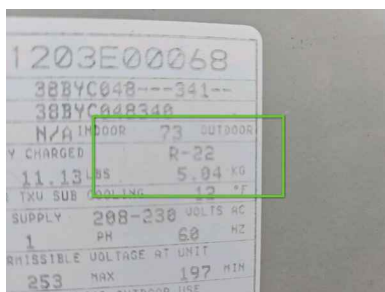
Label at condenser unit
