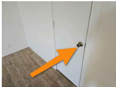
Door to downstairs half bathroom
