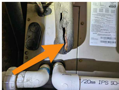
Front of HVAC unit
