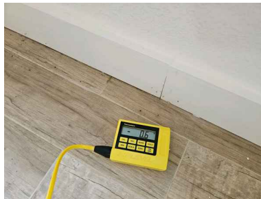
Below middle window at back of house
