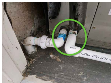
At HVAC unit
