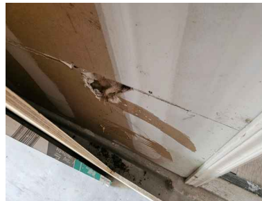
Various locations in garage
